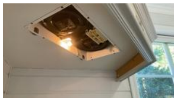
Mnaglene filter oppunder ventilatoren.
